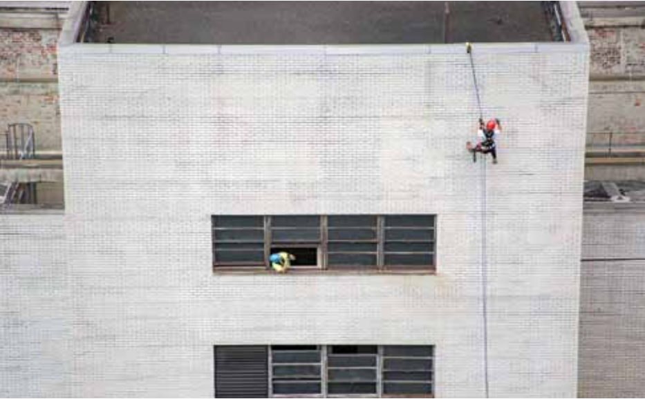
GOES WHEREVER A SPIDER CAN: inspecting a facade by rope (left) and with a drone (below).
